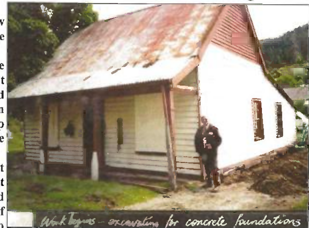
Work begins - excavating for concrete foundations. The Williams Cottage, with Ray Clarkson, one of the trustees, was built in 1864 and is Queenstown's oldest remaining house. It was threatened with demolition in the 1980s. Photo: Lakes District Museum
